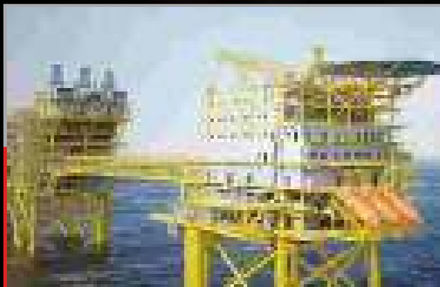
OFFSHORE LQS SKID
